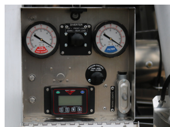
GAUGES, LIGHTS, WEIGHT SCALE, SALCO CONTROL CABINET
